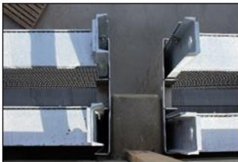
Bolted to Sump Wall
