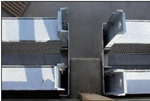
Bolted to Sump Wall
